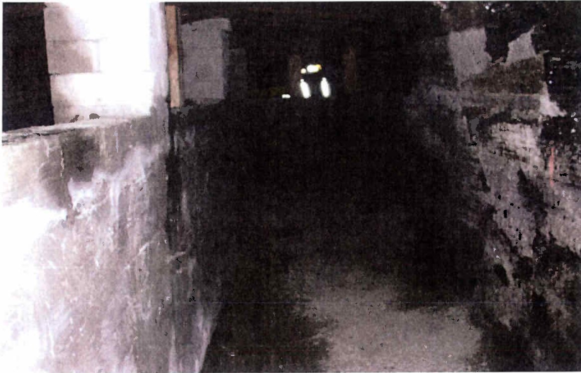
Photo 13: Chamber constructed to impound water against mine rib during preliminary testing at Mine 84.
